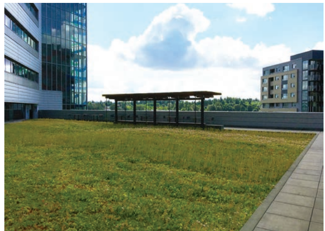
Bellevue City Hall - Bellevue, WA - renovation of roof deck, (built in 2005, renovated 2015)
